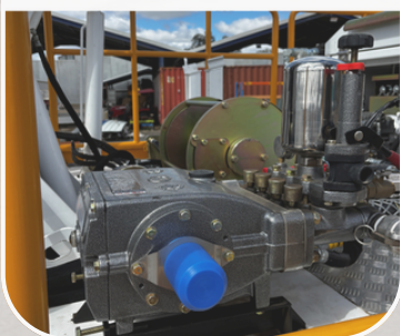
140LPM WATER INJECTION PUMP
